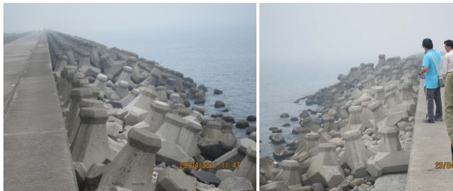
Figure 3. Armoring blocks scattering on the seaward face of the seawall (29th April 2011).
